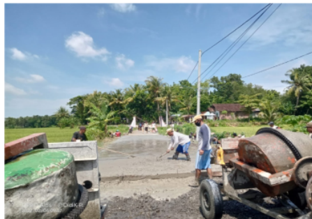
Figure 2. The construction process of the corblok road with PKTD Donotirto Hamlet RT 1
